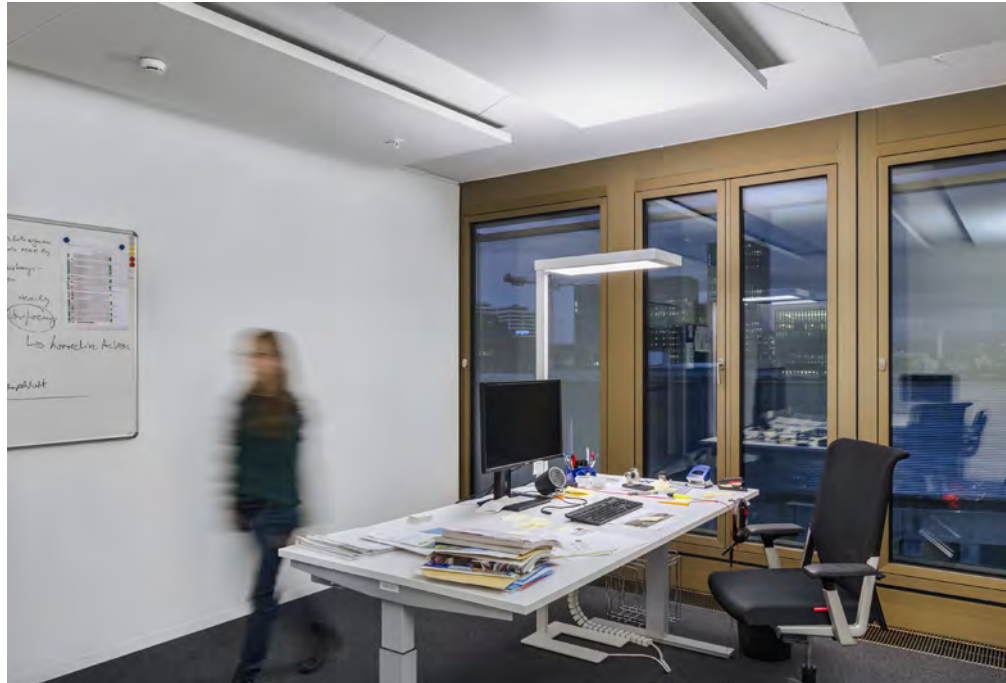
For the showcase, Zumtobel provided 19 high-quality EPURIA free-standing LED luminaires – all equipped with an integrated presence and brightness sensor and wirelessly controlled via Wireless IoT Mesh based on Bluetooth. In addition, six air quality sensors and a gateway were installed and integrated into the network. Photo credit: Faruk Pinjo
